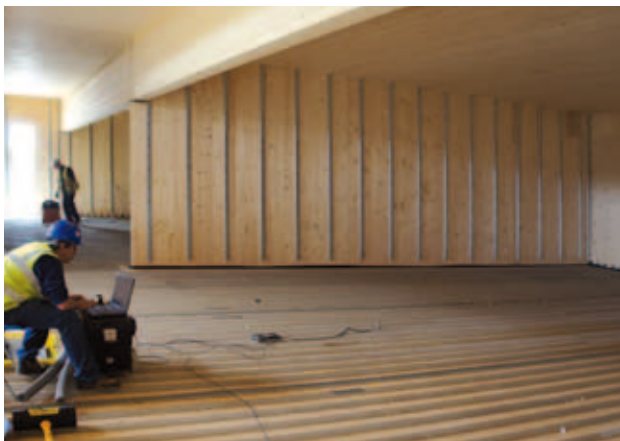
Preparation of KLH® TCC elements for pouring the concrete on site (TimCrete © Ramboll)
